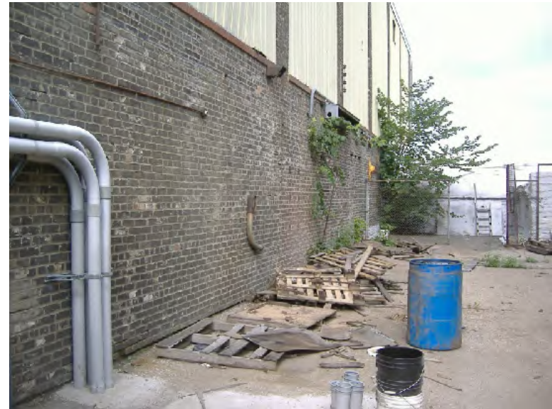
Photograph 8 - Yard of Property in location of former transformer house (view to the west).
